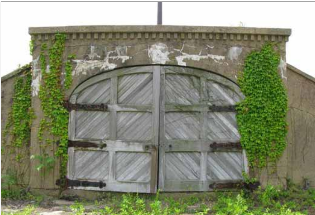
Typical filter bed portal with wood door
