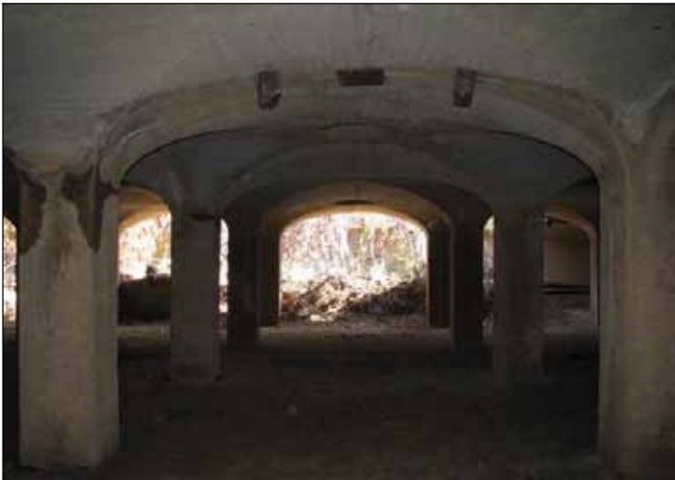
Interior of filter bed No. 24, collapse of eastern cells.
