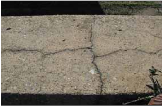
Typical crack in wall of service court
