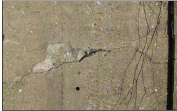
Typical crack in wall of service court
