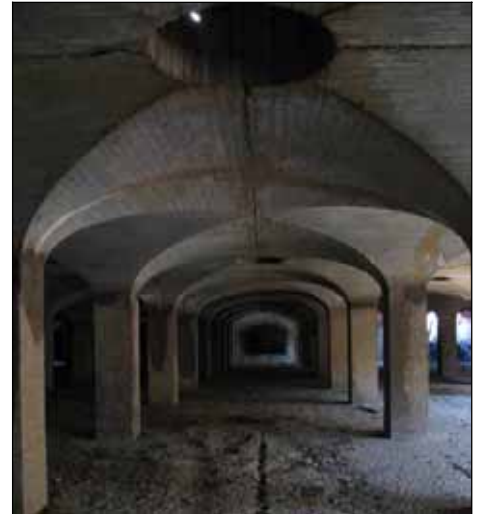
Interior filter bed No. 24
