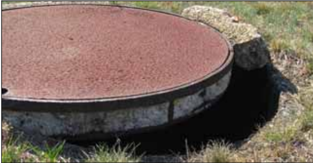
View of inner and outer covers of deteriorated manhole
