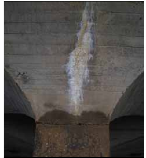
Cracking and efflorescence of concrete structure
