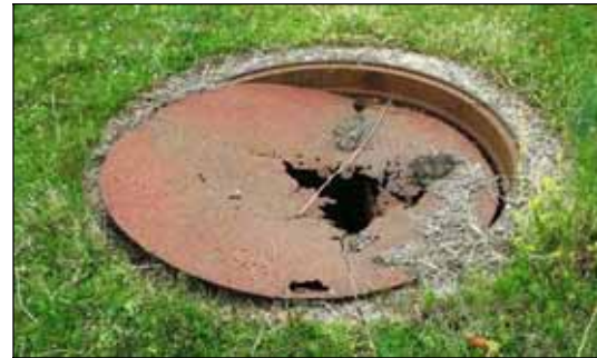
Corrosion of manhole cover
